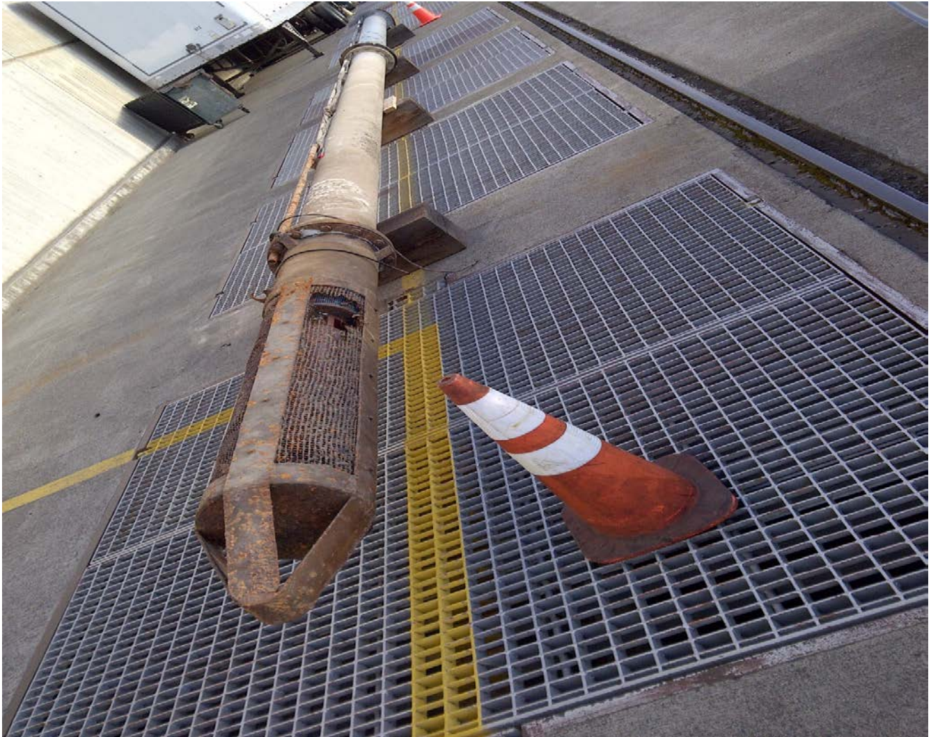
Failed collection channel dewatering pump. Requires new power conduit and screen. Remaining 8 pumps will be removed and inspected for similar problems next winter as funding allows.
